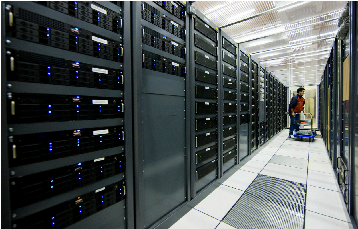
Reuters/Valentin Flaraud – A technician performs maintenance in the CERN LHC computing grid centre in Geneva
